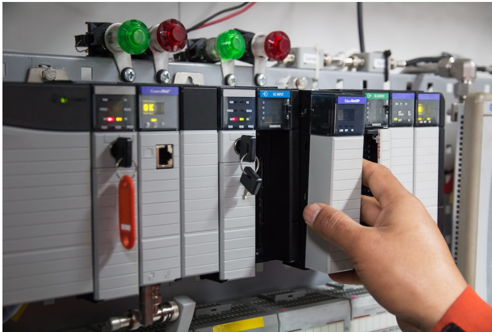
Figure 193 | PLC with I/O Modules
