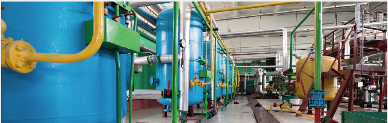
Figure 197 | Inside a Water Treatment Plant
