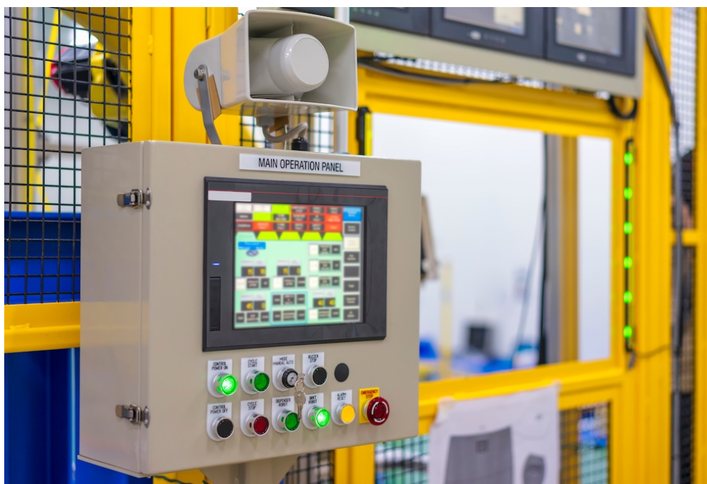
Figure 196 | Embedded Human Machine Interface Panel
