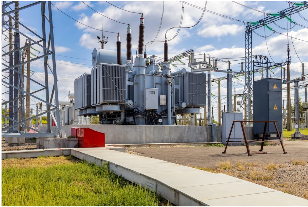
Figure 195 | Electric Power Substation Yard
