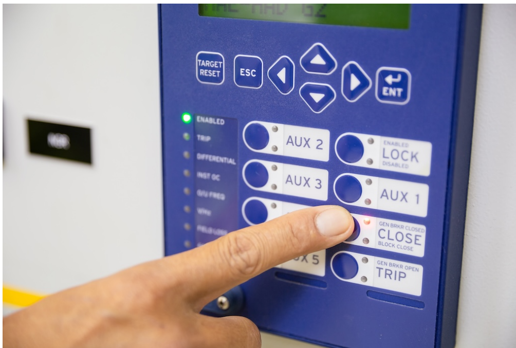
Figure 194 | Protection Control Relay
